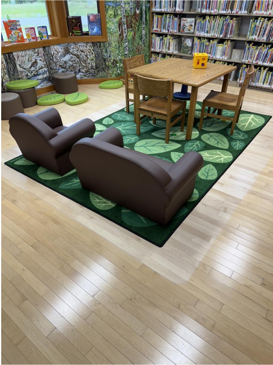
Photo #7: Kids Room discoloration of floor
